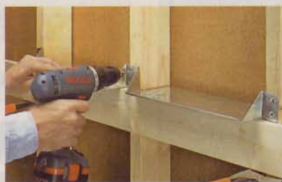
Locate and level a shelf, and then attach it with two screws at each end.
