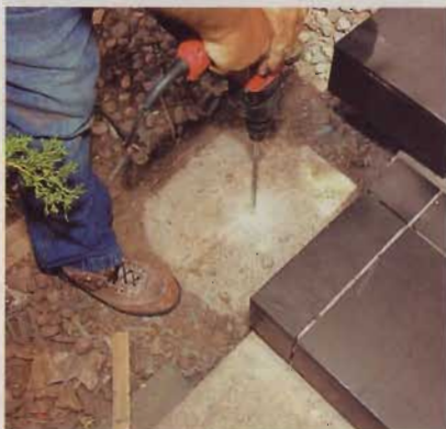
1] After pouring footings for the columns, drill holes to accept steel rebar using a hammer drill and masonry bit.
