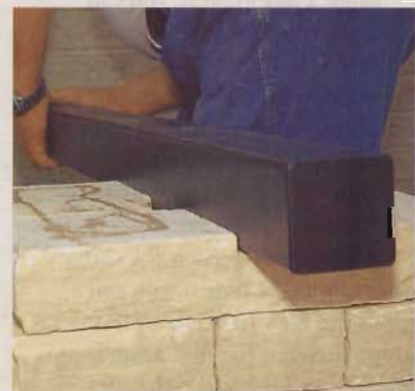
3] Now fit the steel tube in place on the column. A notch cut in the stones accepts the tube easily.
