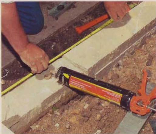
3] One of the best ways to ensure staggered seams is to measure out from the corner, and then cut a stone to fit the space.
