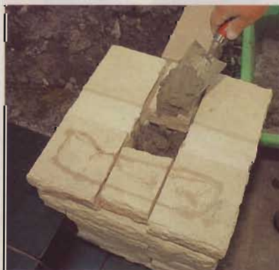
2] Before adding the steel tube, insert the rebar, and fill the center of the column up with concrete.
