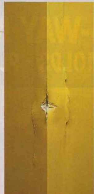
Severe corner damage like this requires a new piece of corner bead. That means you'll need to cut out the existing piece with a hacksaw ( left ).
