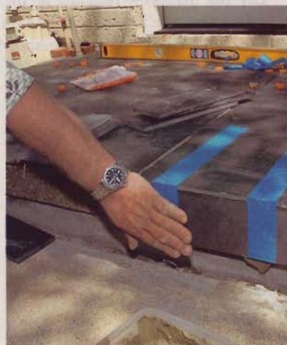
5] Then press the edge tiles firmly into place, and secure them with masking tape until the mortar sets.
