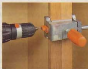
Use the guide to drill into the edge of the face frame.
