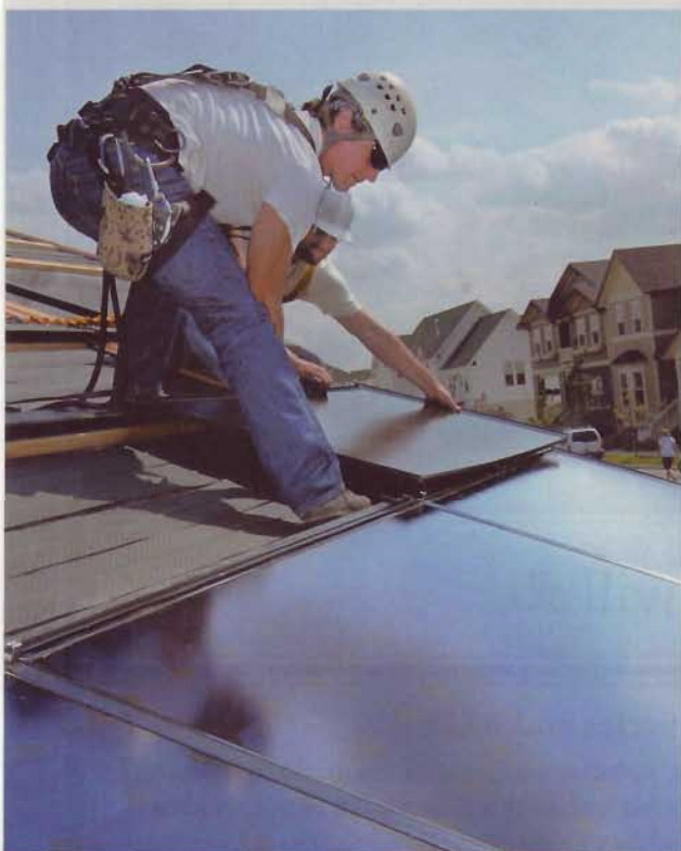
Students install rooftop panels that will take advantage of solar power to produce electricity.
