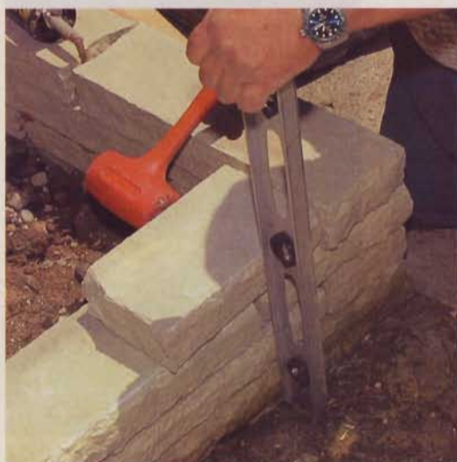
5] To make sure the wall stands straight, hold a long level along its outside face. If necessary, tap the stone lightly with a mallet to bring it into position.
