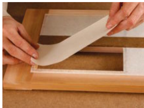
An invisible repair. Apply a new section using the same paper, and the panel will look as good as new.
