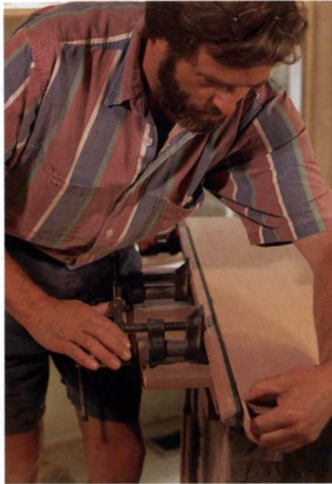
If the edging is 1/8 in. wider than the plywood, then the alignment is not crucial. You can trim the overhang later.
