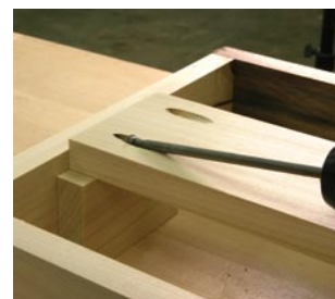
The catch rail for the top unit rests inside the end rails. To keep the rail from sliding downward as the screws are installed, rest the piece on a block cut to the correct size.
