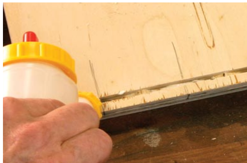
Practice getting the right amount of glue in the slot. You want to coat the surface of the plate without having excessive glue squeeze-out, or introducing too much moisture in the interior of the joint.
