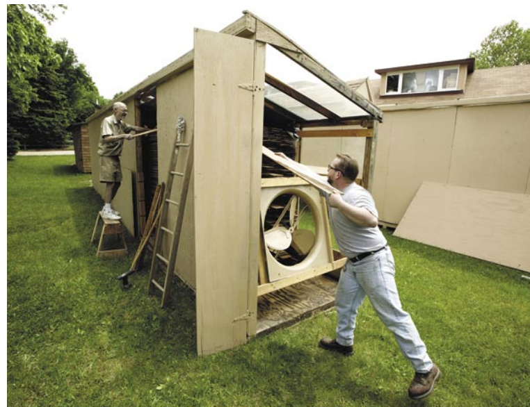
Here, we replace the fan, which will be plugged into a receptacle whose power is controlled by a thermostat. The end wall is closed by using drywall screws to secure the door and the main end panel.
