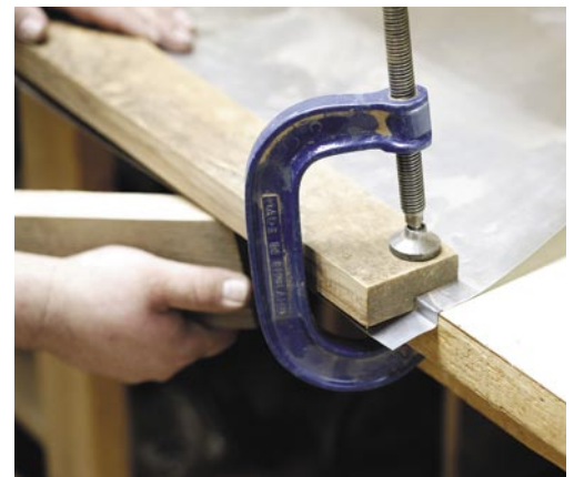
Bending the aluminum flashing used in the 1/4" ledge on which the window wall glass will rest. Step one was to make a right angle in the flashing. Here, the final bend is facilitated by a board with a 1/4" rabbet sawn in it and clamped to the bench.
