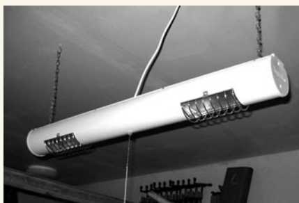
A Regent 300-watt halogen shop light suspended above my table saw provides bright, shadow-free lighting at the saw blade. The housing is 36" in length and features diffused tempered lenses, safety screens and a pull-string on/off switch. This lamp augments the workshop's fluorescent lighting.
