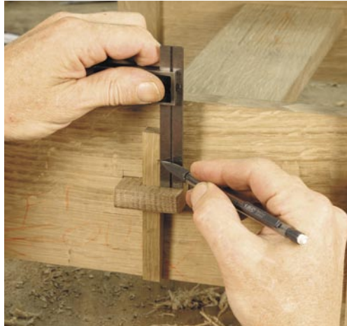
As the tenon key is fit, the length above and below the through tenon changes. I leave the key long and mark the length once I have a good fit.
