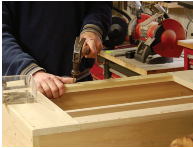
Carefully drive the nails that attach the face frame. (If you miss and ding up your stock, don't despair. Just spoon a bit of water onto the ding. As the fibers swell to accept the water, the surface of the wood will return to its original configuration.)
