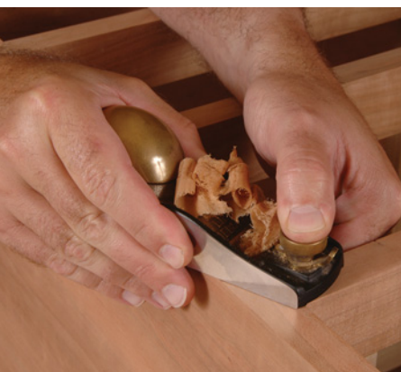
A standard-angle block plane with a 55° cutting angle is useful for leveling the joints. This high cutting angle reduces tear-out in some tricky woods.
