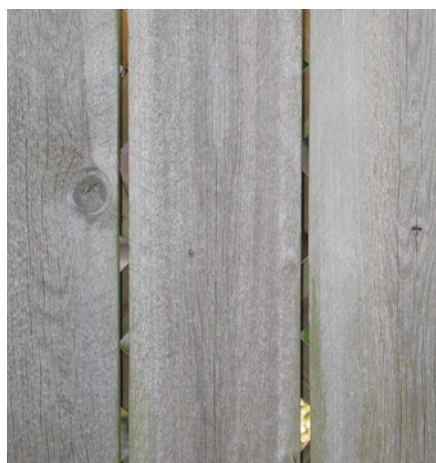
The combination of sunlight and rain causes wood to turn silvery gray. If you like the gray color, and you aren't having other problems, you can leave the wood unprotected. The grayed surface is very effective at blocking further degradation below. UV light erodes wood at only about 1/4" per century.
