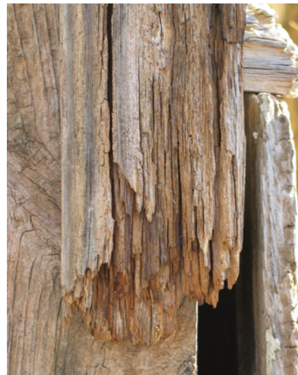
Rot is very destructive to wood, as is obvious in this photo. Pressure-treated wood and the heartwood of redwood, cedar and a number of exotic woods including teak, mahogany and ipe resist rot. A wood preservative that is not pressure-injected is fairly ineffective at preventing rot on non-rot-resistant woods.
