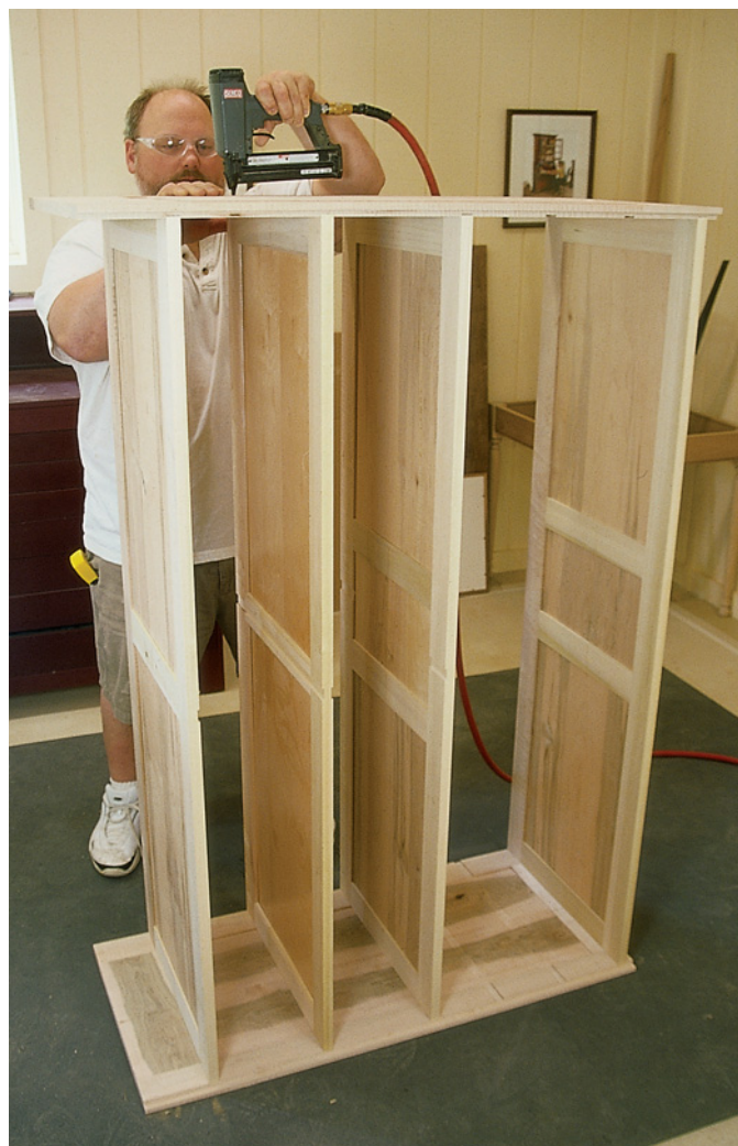
When all the dados and grooves are complete, you're ready to assemble the carcass. Glue is important, but I find a good 16-gauge finish nail goes a long way to holding everything together. Notice that the lower horizontal dividers have one center rail, while the two upper dividers have two. These correspond to the vertical dividers.
