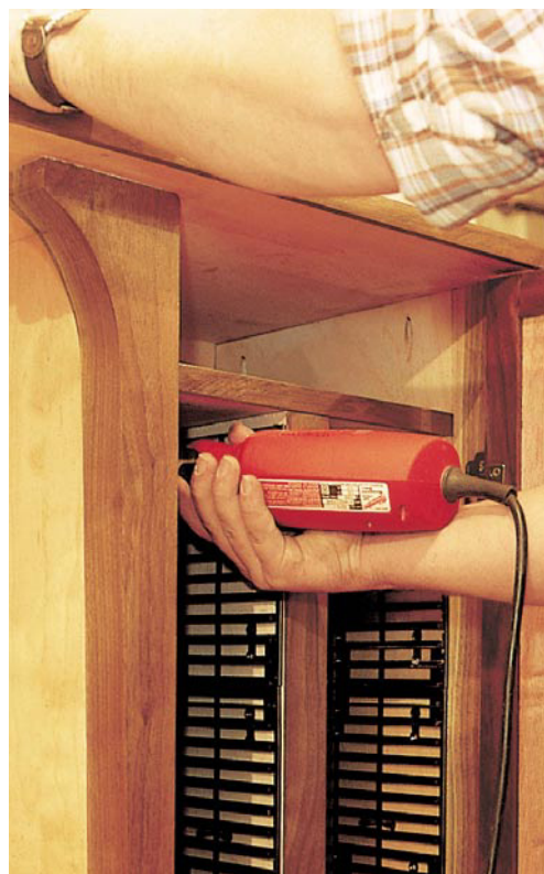
Installing the CD racks is tight work, so the close-quarters right-angle drill came in very handy. Too bad I had to borrow one, but a trip to the tool store will fix that shortly.
