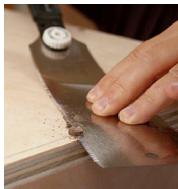
Before attaching the second side, it makes sense to cut the dowels on the first side flush to the surface. I used a Japanese flush-cutting pull saw that has teeth with very little set to them, reducing the chance of scratching the cabinet side. By applying pressure on the blade to keep it flat to the cabinet surface, I further reduced the chance of scratches. Do a little sanding, then flip the cabinet over and attach the second side, then the front.
