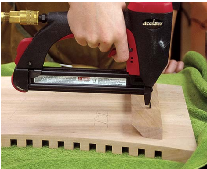
Here you can see I'm attaching the French cleat to the back of the curved wall-hung rack. This cleat, along with another block of wood that's attached further down the piece, will make the rack look like it's floating on the wall once hung.
