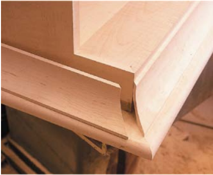
With the upper case flipped over, you can see the top and sub top extending beyond the cabinet, with the filler, top cornice moulding and crown moulding ready to be put in place.
