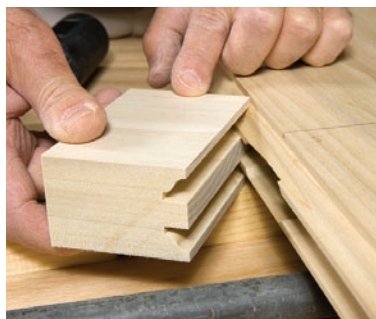
Seat the lock-rail to the middle mullion joint by applying a clamp momentarily. A coped scrap is valuable as a clamp block to protect the stuck edge of the lock rail.
