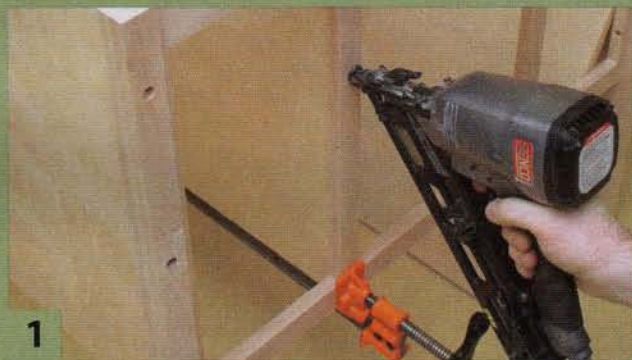
1 Begin building the router table by making the base. Construction is quite simple, using just screws, glue, and a nailed-on face frame in front.
