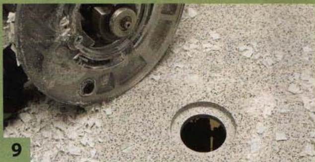
9 Enlarge the opening by using a series of rabbeting bits and pattern bits. A rabbeting bit leaves a ledge around the hole making it perfect for fitting an insert.
