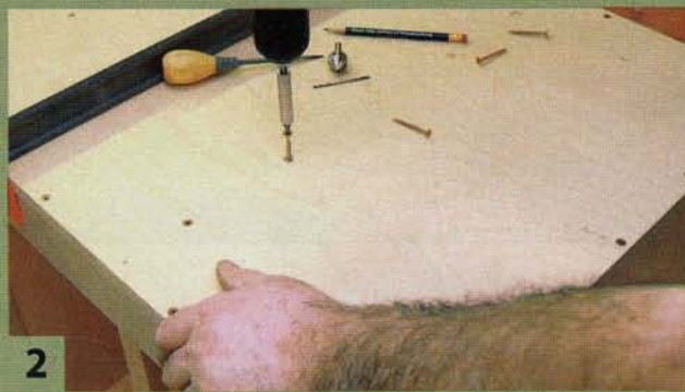
2 Attach a plywood sub-top to the base. The subtop prevents the base from racking. It also supports the working top which is made from 1/2" thick solid-surface material, such as Corian or Avonite.
