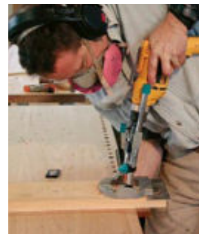
With so many spindles, consistency was crucial. A jig helped Clark space the holes and drill them at the proper angle.
