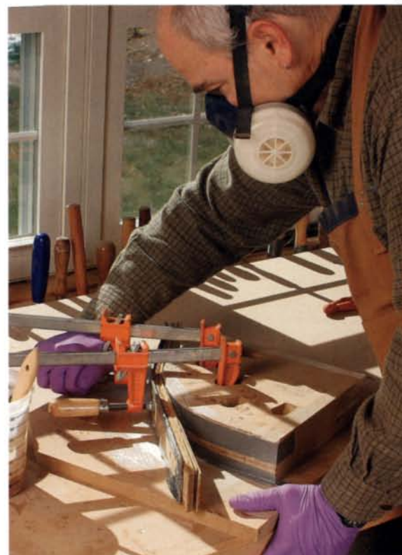
Clamp from the center out. When clamping the glued-up lamination, apply the clamps sequentially from one point outward.
