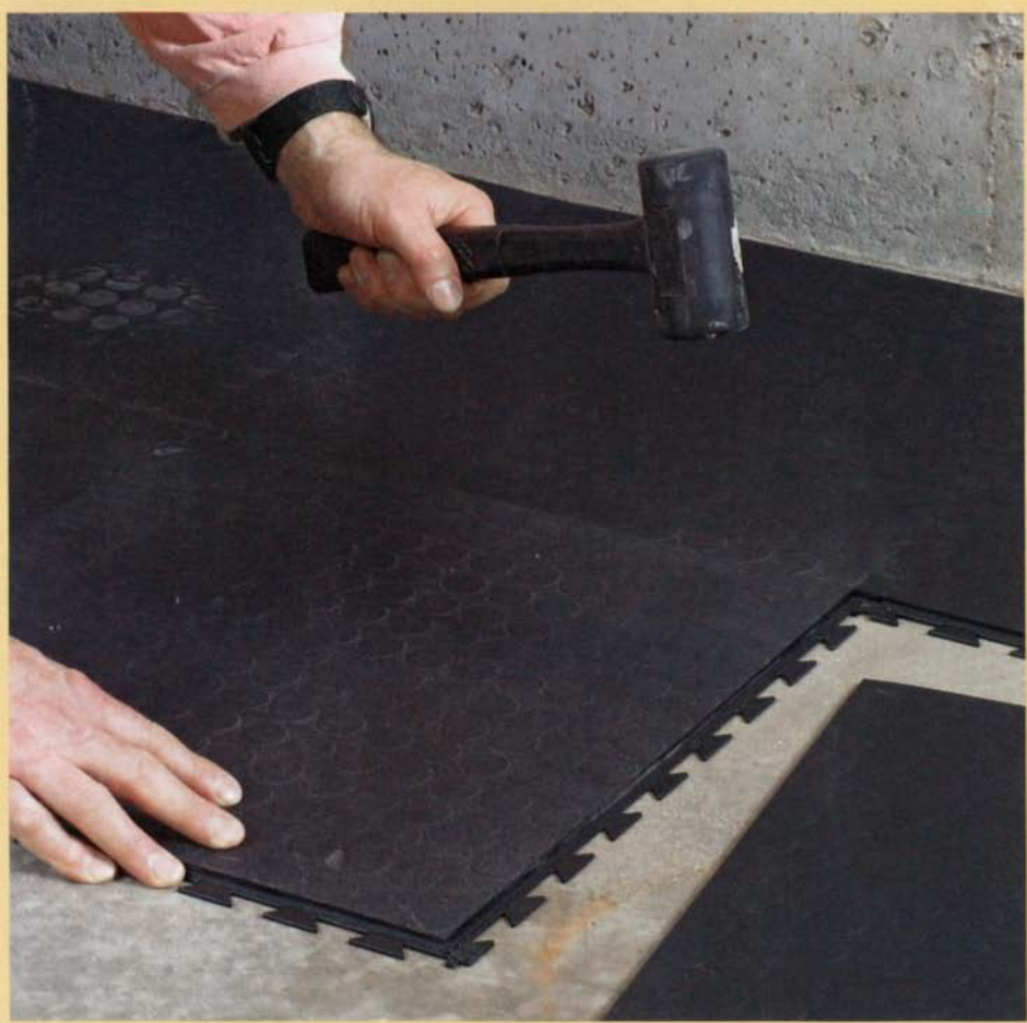
The tight interlocking tabs are joined easily with a mallet. Knock the interlocking edges into place with a rubber mallet for a snug, flush seam.
