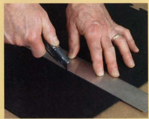
Trim the tiles with a utility knife and a straightedge. PVC tiles are thin enough to be cut to size with a standard utility knife.
