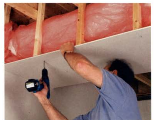
Skin the frame with drywall. Sheets of gypsum board add mass to the chased opening and deflect much of the airborne sound.
