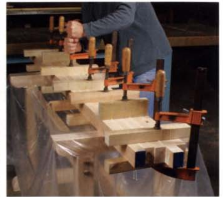
Use cauls to keep the slab flat. Wrap them with clear tape for easy cleanup. Snug them down first, then clamp across the width.
