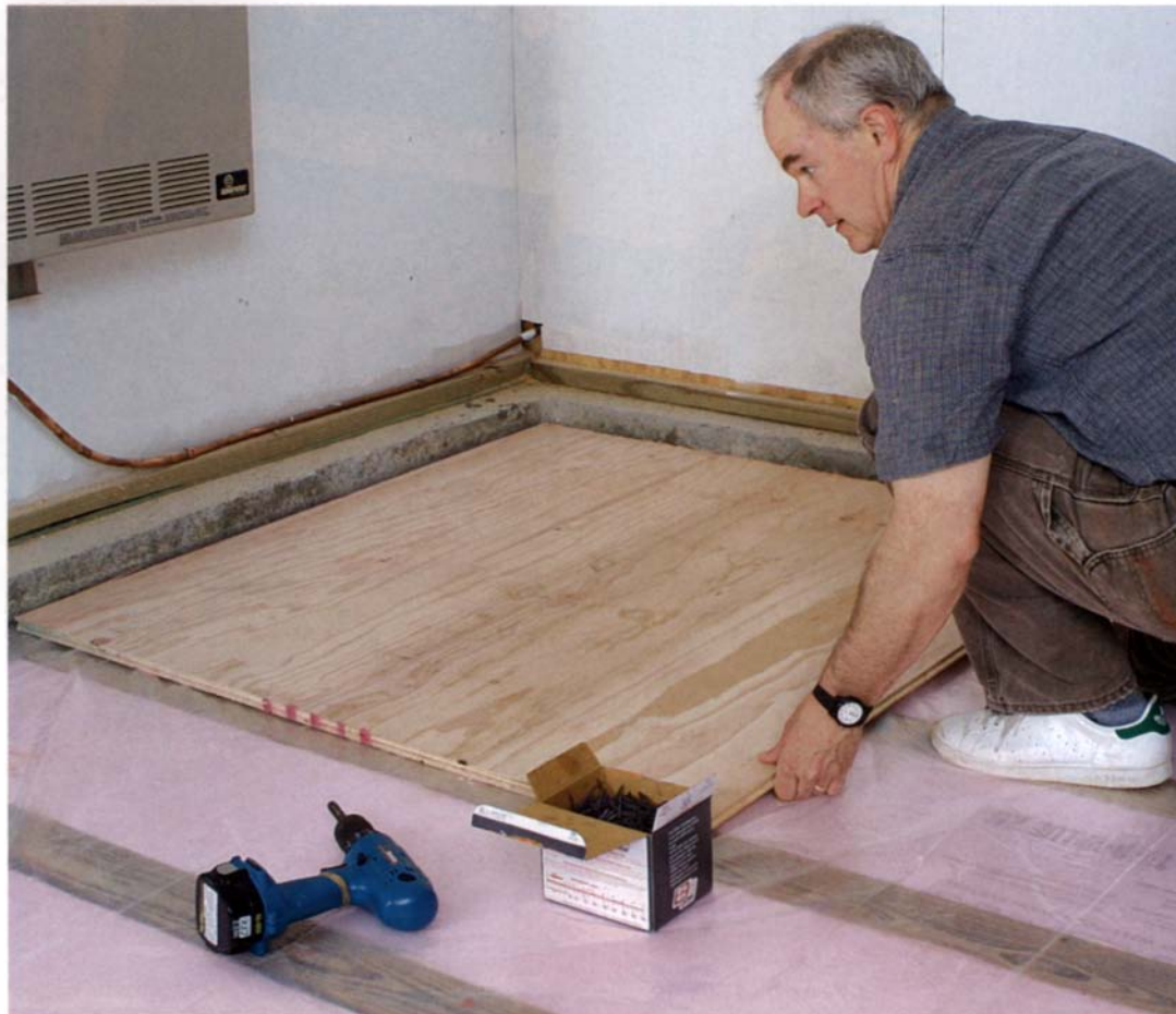
Get the first piece right. Take your time placing the first plywood sheet because all of the other pieces will follow its course. Be sure to leave a ½-in. gap at the walls around the perimeter to give the plywood some room to expand.
