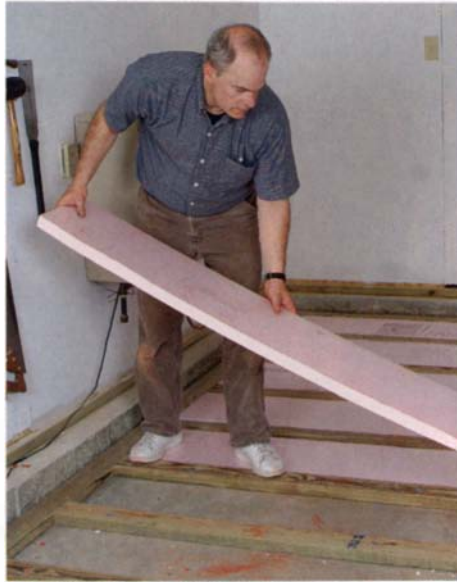
Insulation to keep your toes warm. In colder climates, place rigid insulation between the rows of sleepers.
