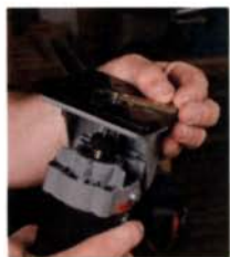
Set the depth of cut equal to the thickness of one hinge leaf. A laminate trimmer makes quick work of routing the mortise, leaving little waste to be cleaned up with a chisel.
