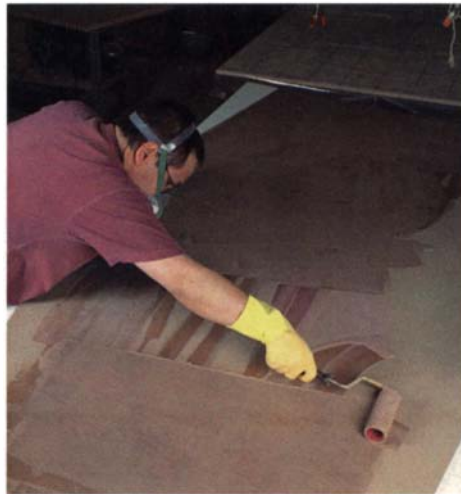
Don't spare the glue. A liberal amount of urea resin glue applied with a squeegee and roller guarantees a rigid bond at the glueline.
