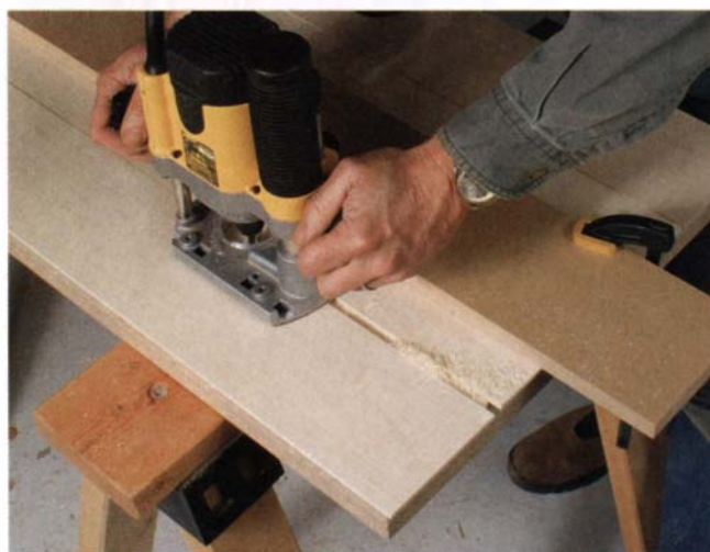
Rout the joint. To clean up any gaps, a router and edge guide are used to cut a shallow groove centered on the long joint.
