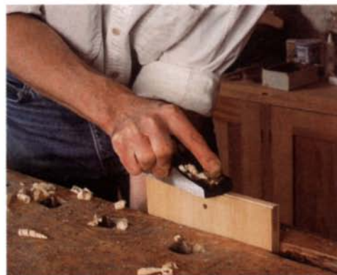
Finishing up. Insert the pins, take off the clamp and plane the cleats flush with the ends and edges of the plank.
