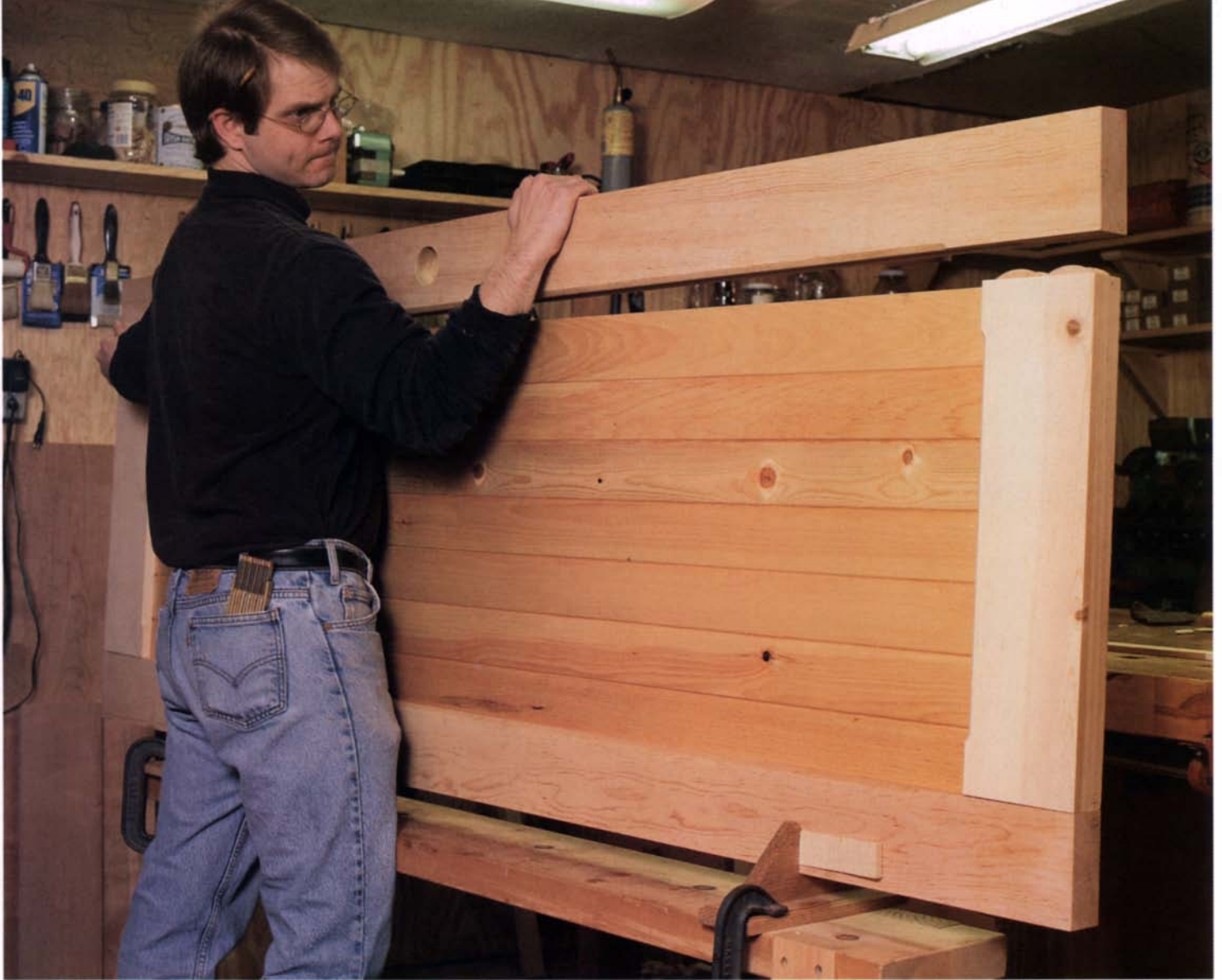
When everything is square. Work blocks clamped to a sawhorse hold the door steady while it's dry-fit. Using a polyurethane glue allows plenty of time to make sure that everything is flush, square and aligned. Just remember to mist the biscuits with water to help the glue cure properly.
