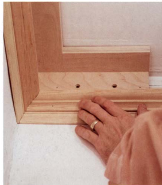
Coped joints are cleaner. The first two layers of this cornice, an inverted baseboard and a bed molding, were installed with coped joints at the inside corners.
