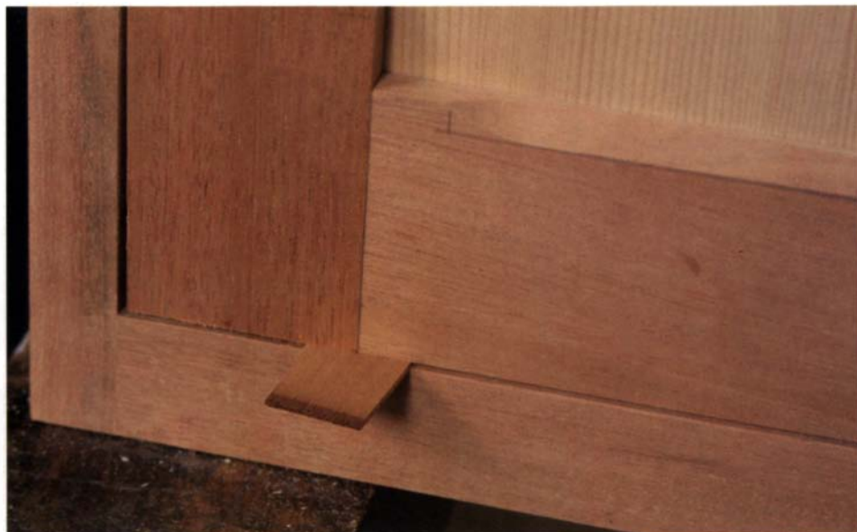
Dry-fit with \frac{1}{16} -in. shims under the door. Check and adjust the hinge stile next and the top after that. The joint between the doors is the last edge to be fit.
