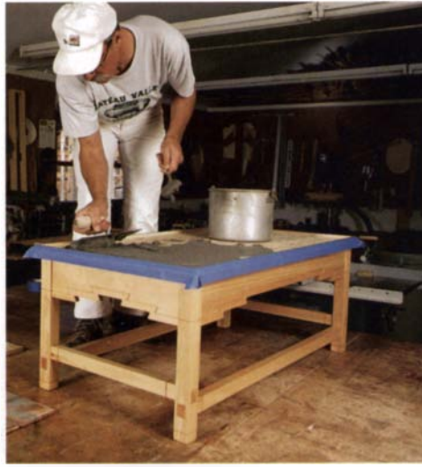
Leveling the mortar— Using a screed board, Jordan makes sure the mortar is an even thickness across the substrate.
