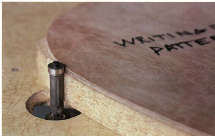
For fair, twist-free panels, ribs must be of consistent size and shape. McCaffrey marks out a template for the mating half of a form (above middle). Tacked to a particleboard blank, the template guides on the pilot bearing of a flush trimming bit, cutting the blank to final size (bottom).
