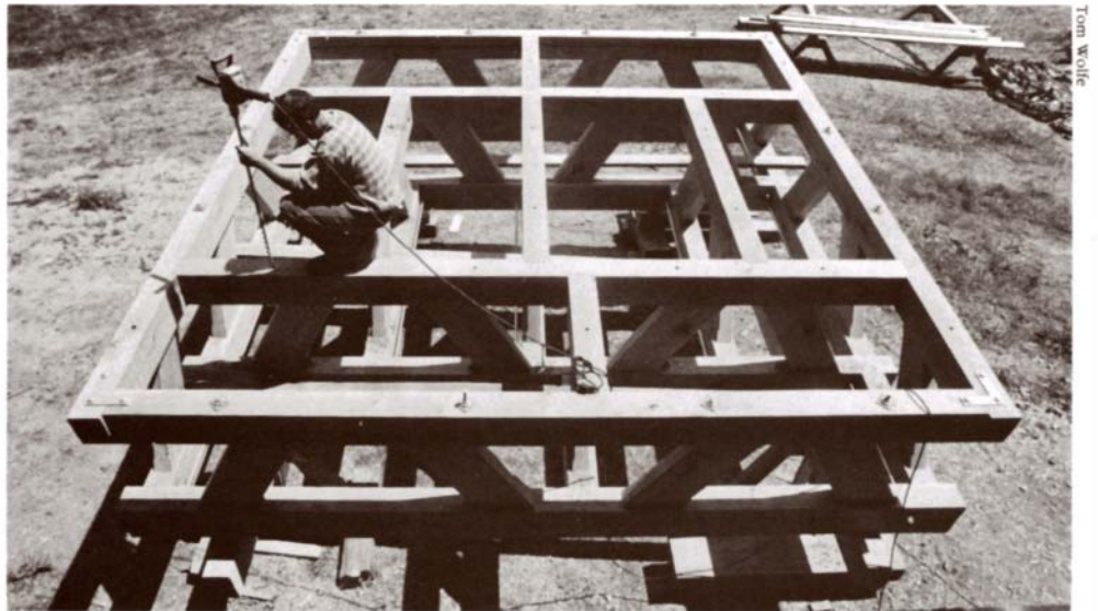
To resist the enormous racking forces of three tons of swinging bells, timber framer Ed Levin built the Old North Church's new bell frame of heavy white-oak beams. The beams are mortised and bolted together.
