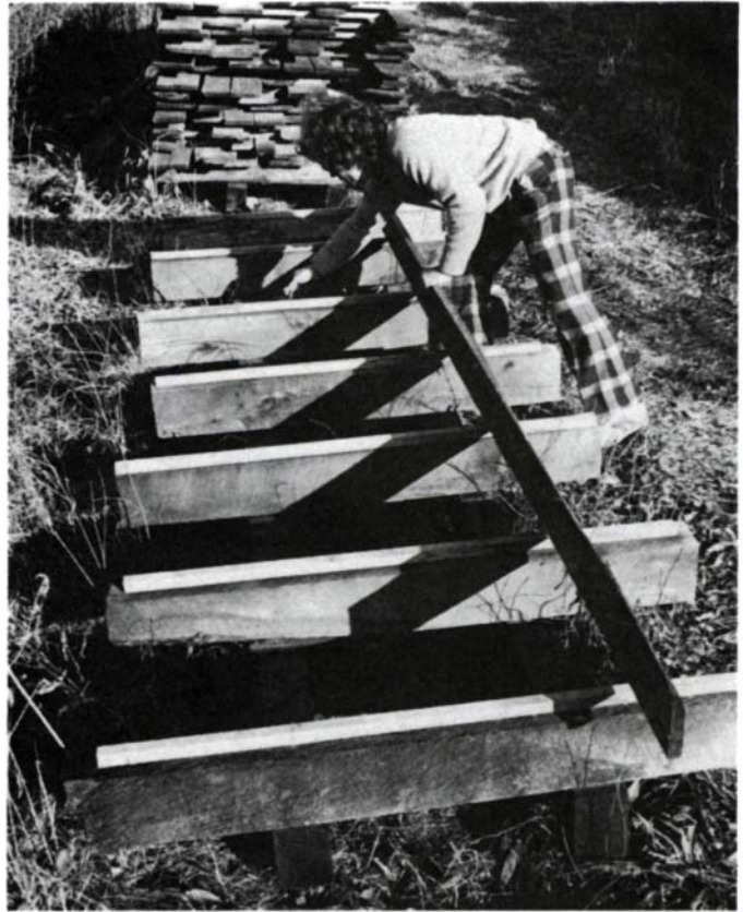
Paul Fuge makes sturdy foundations for his lumber stacks. He checks alignment of bolsters with a long, straight board fresh from the sawmill. To build a foundation with lighter stock, shore up with more concrete blocks or make a smaller pile.
