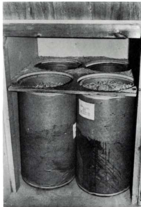
Shavings and heavy particles are collected in four barrels at the bottom of the drop box. The baffle board on top prevents waste from falling between the barrels.
