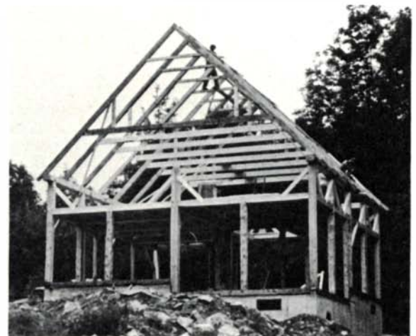
Framing diagram (above) and first floor plan (left) of a typical two-story house in New England of the late 18th century. The contemporary frame in the photo follows the same scheme, except that its second story posts are reduced to a knee wall. This permits almost as much usable space, with considerably less timber.
