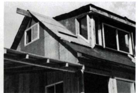
Details at left show rafter joinery, green-oak decking. Windows are installed after framing is sheathed in particle board and covered in tar paper, above, then exterior is finished with white pine boards.
