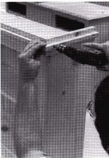
11-13 Attach the angled cleat to the reveal with 1 1/4-in. drywall screws. The cleat and the reveal are both 3-piece assemblies with mitered corners.
