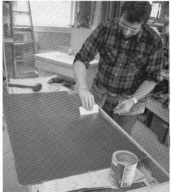
6-10 With a scrap piece of laminate, I spread contact cement evenly over the underside of the plastic laminate. Give the particleboard and oak trim the same treatment.
