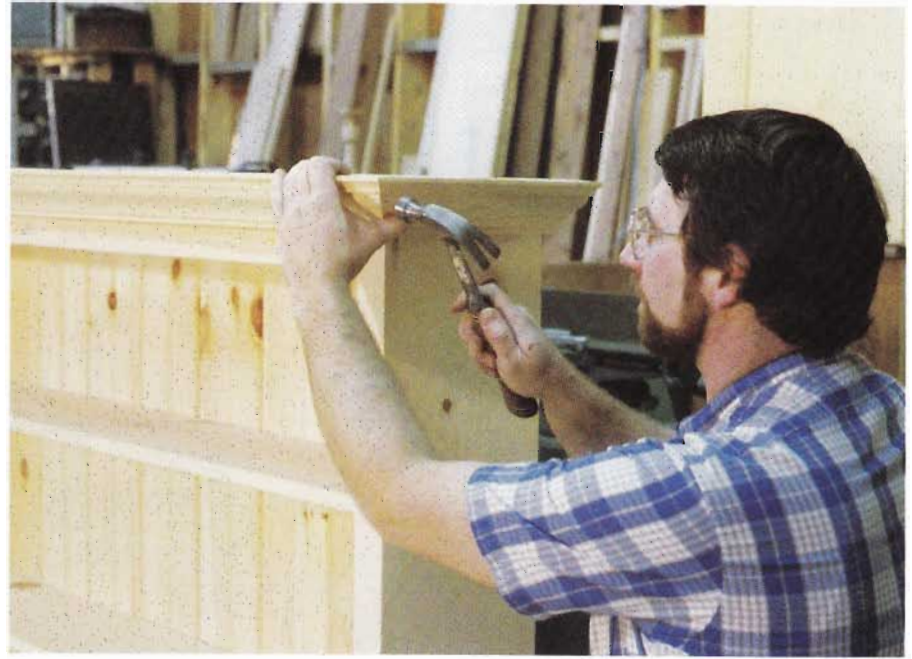
11-15 I use 4d finish nails to pull the molding's miter joints tight while the glue sets. Nails should be set carefully and then filled after finish has been applied.
