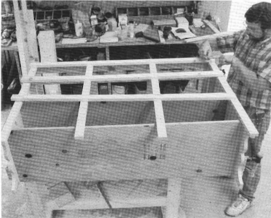
11-5 Accuracy is crucial in laying out the lap joints in the face frame. The surest way to get the layout right is to mark up the pieces while they're in place on the front of the base.
