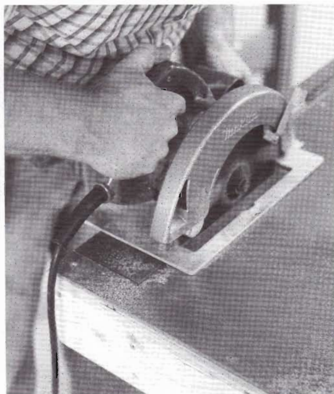
2-9 Cut out the tailstock opening after screwing the top to the frame. To cut the long side of the opening, you'll have to make a pocket cut, carefully lowering the blade down into the top. Finish cutting out the corners of the opening with a hand saw.
