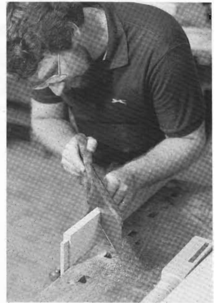
3-8 With the rail clamped in the workbench, I use a back saw to cut out the end of the brace at a 45-degree angle. A second end-cut frees the brace.
