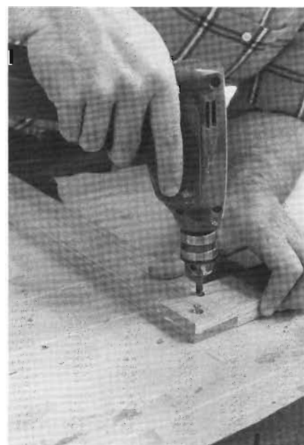
1-8 The lap joints at the corners of the face frame are glued and screwed together. Drive a pair of #6 flat-head, 1/2-in. screws into the back of each joint to pull it tight.
